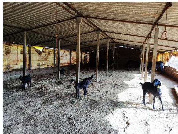
Goats are maintained in spacious semi open shed with GI roof in Zharwad
